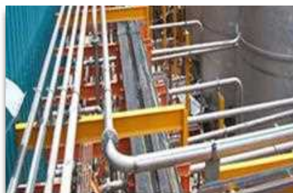
MS And SS Pipelines
